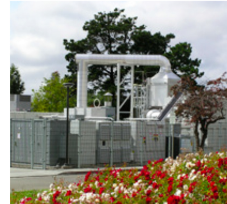
DFC@1500 EU MCFC-Fuel Cell Power Plant 1,4 MW; 20 kV; 50 Hz
